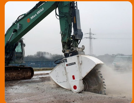
The central concrete slab located between the two hollow box sections of the bridge was also cut using the cutter wheel and then cut into smaller sections using a concrete saw.
