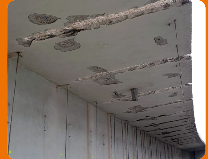
A segment of the western cantilever arm. After cutting through it longitudinally using a concrete saw it was separated from the main section using a crane.
