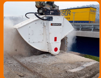
The cutter wheel is used to cut through one of the cantilever arms on the old bridge. Behind, traffic flows over the river Saar on the new bridge.
