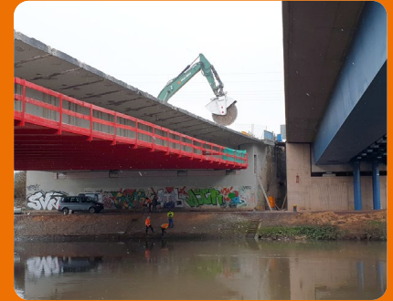
Bridge demolition at the Saarlouis autobahn junction: The new bridge takes the road BAB 8 over the Saar River (right). Demolition experts Max Wild start demolition of the old bridge with the aid of a KEMROC DMW 220 cutter wheel.
